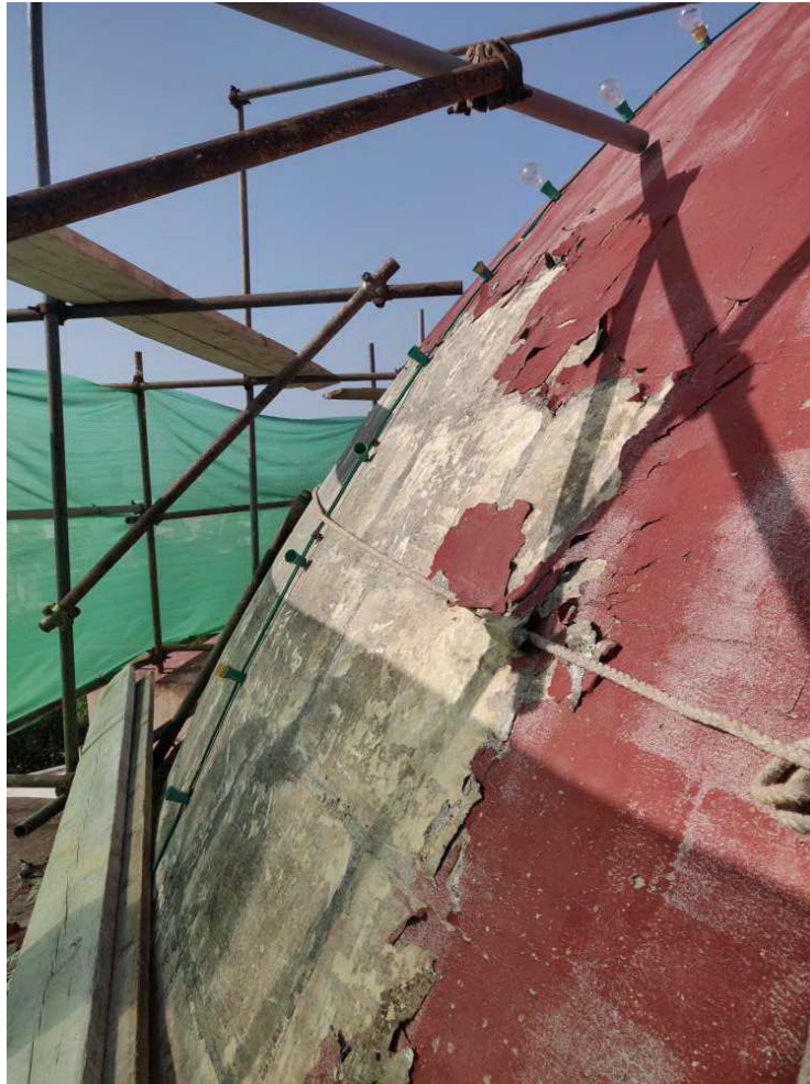
Plate 5: The peeling paint layers exposing the masonry dome underneath.
